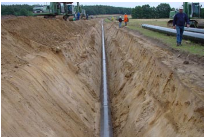
Fig. 6.1. Trench in unstable soil
