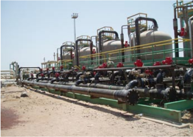
Fig. 7.1. Aboveground pipe system
