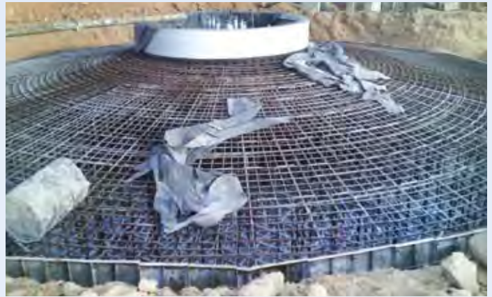
Foundation work for Wind Mill project of Railway Energy Management Company Ltd (REMCL), under installation
