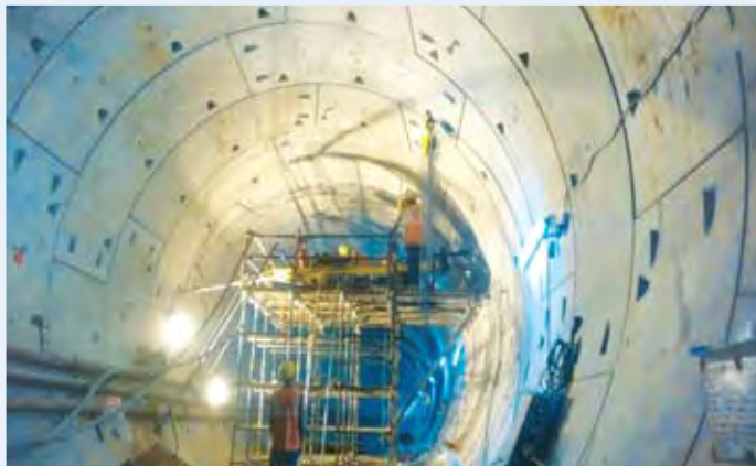
Cross Passage CP-01 – Pipe Roofing Work in Progress b/w Lajpat Nagar – Vinobapuri Tunnel (CC-24), Delhi Metro
