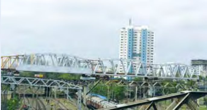
Launching of open Web Girder across Railway Tracks for Monorail at Wadala, Mumbai under Supervision of RITES
