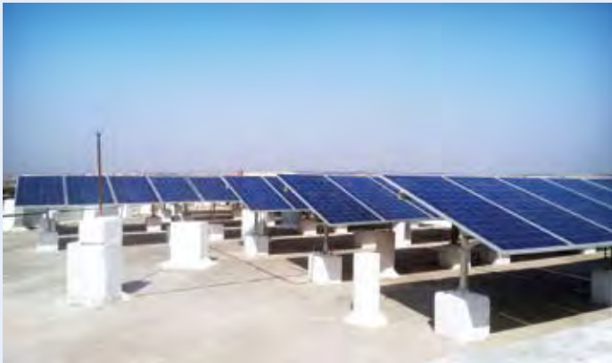
Promoting renewable energy: 40 kWp Solar Power Plant at Central University of Gulbarga, Karnataka
