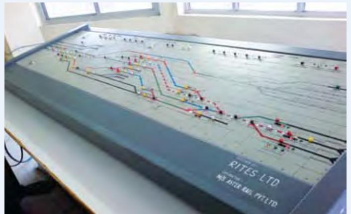
Route Relay Interlocking at NTPC, Vindhyachal (MGR)
