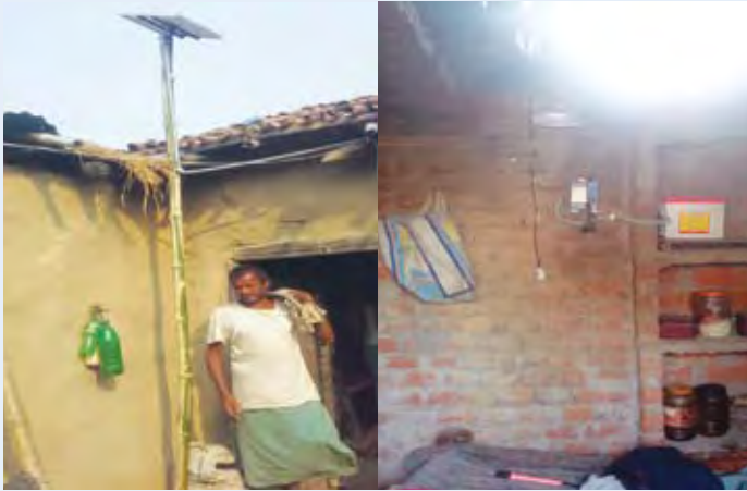
Sustainable Development: Reaching out to villages through Renewable Energy, Distt. Gaya, Bihar.
