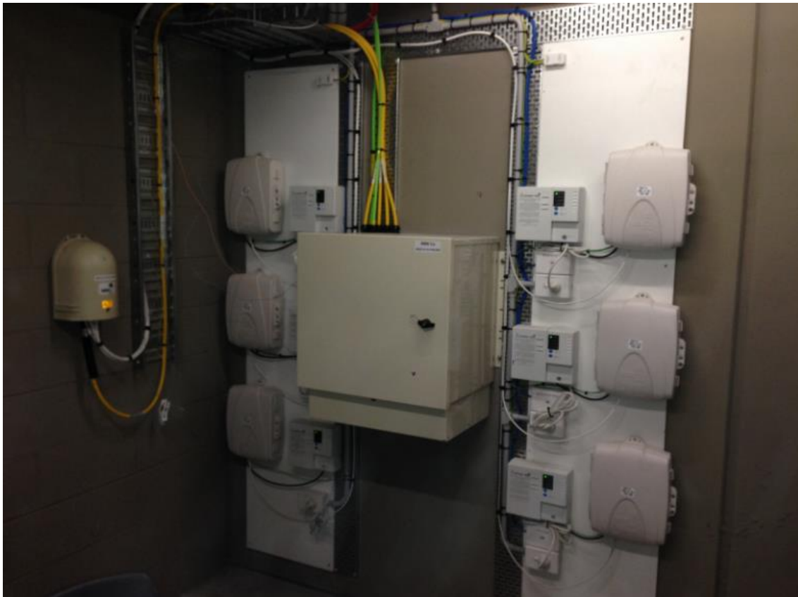
Figure 13. Example of typical communications room
