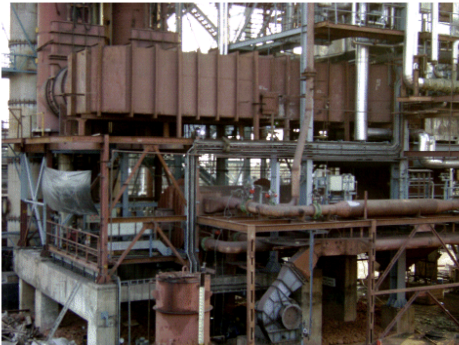
A closer view of the plant
